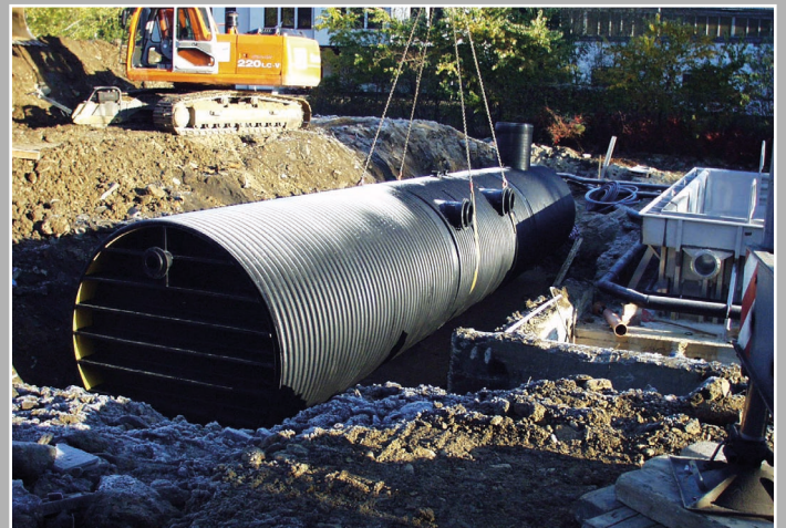
Retention tank of a public swimming pool, DN/ID 3000 mm
