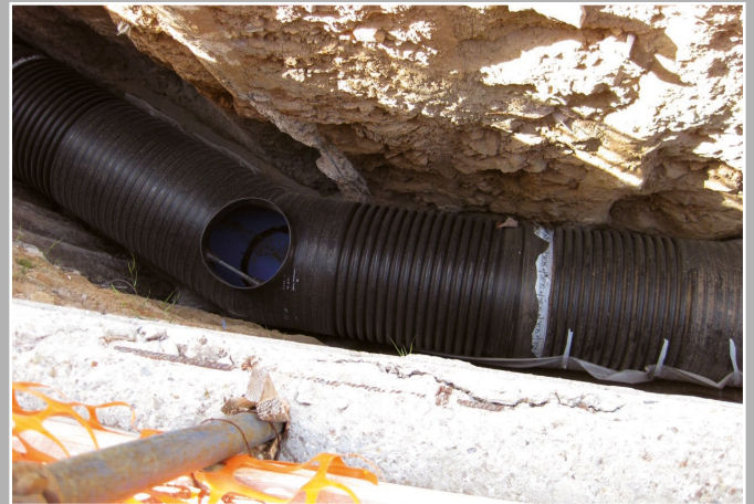
Storm drainage line with integrated manhole
