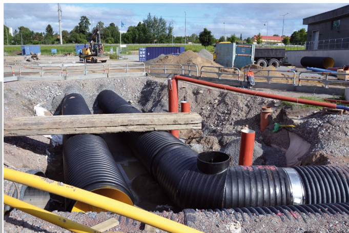
Fire fighting water tank
