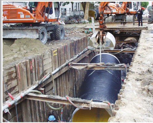
Sewer pipeline DN/ID 2000 mm
